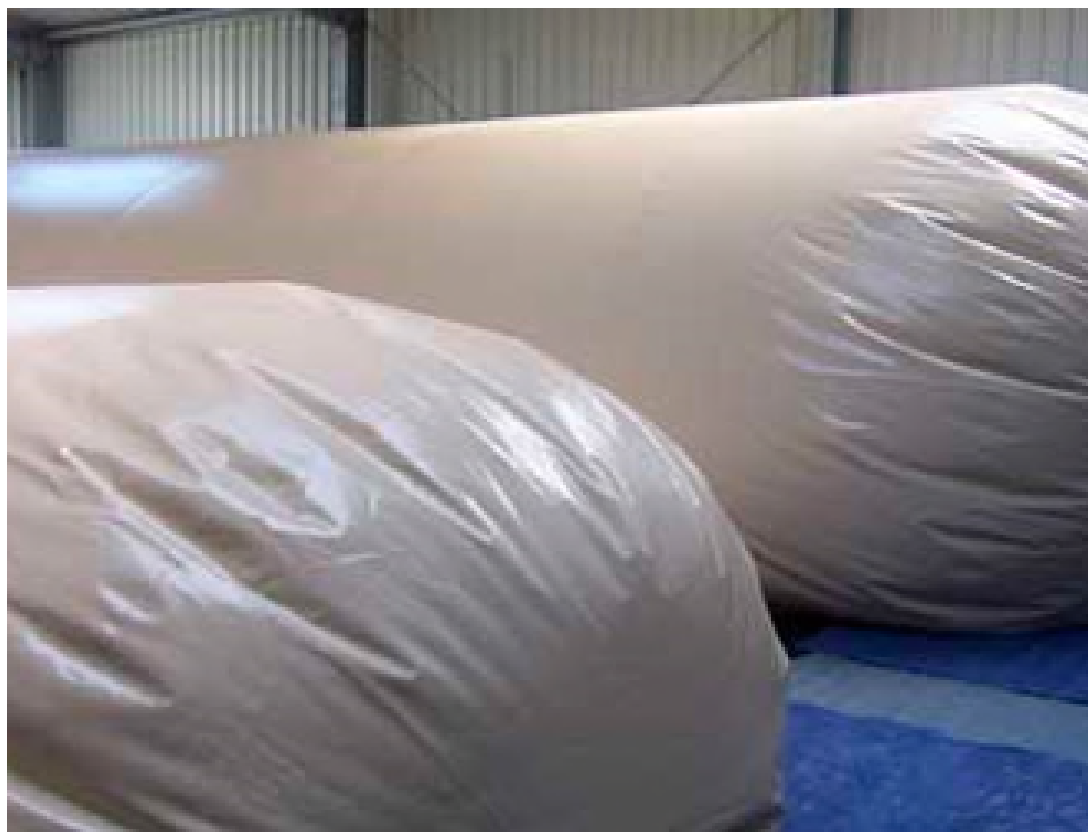
Figure 3-3. External Biogas Holding Bags
