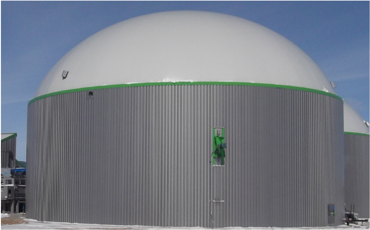
UW Oshkosh Biodigester at Rosendale Dairy – photo by David Palmer
