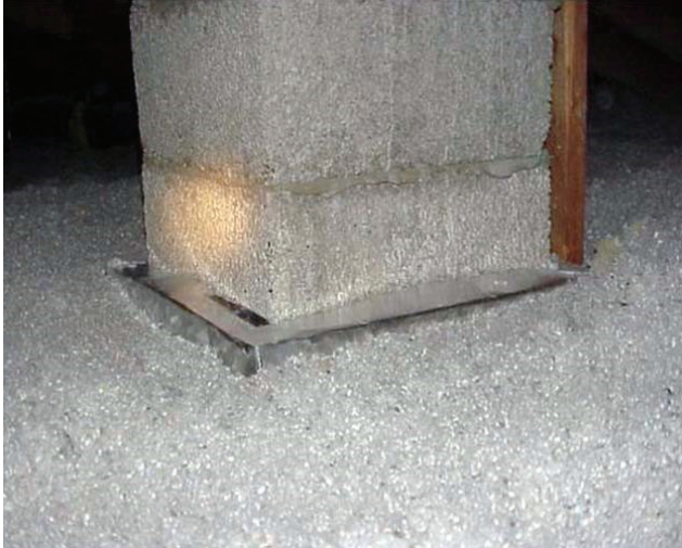
Attic insulation dammed away from chimney
