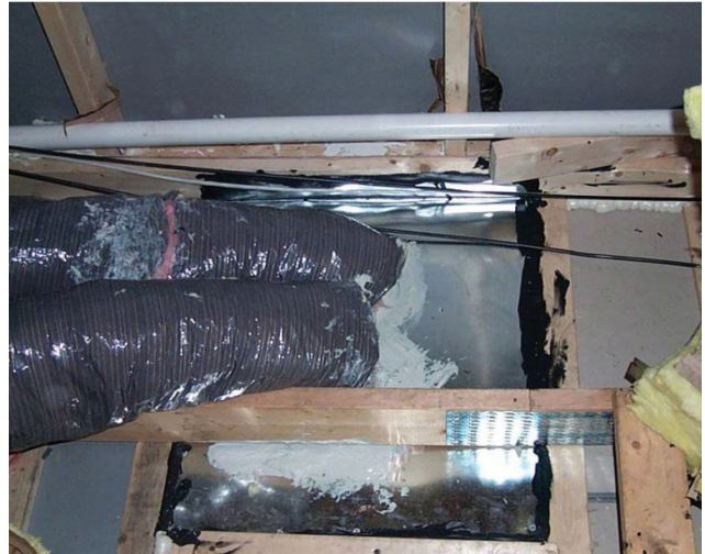
Open attic chase sealed with sheet metal, duct mastic and acoustical sealant
