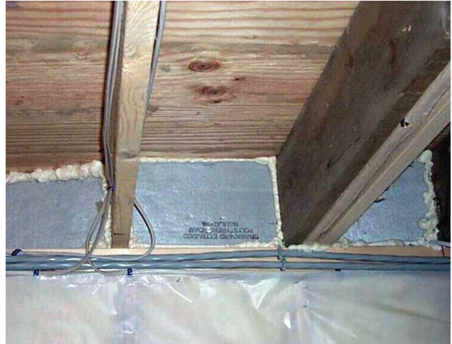
Rim joist insulated (and sealed to sill) with foam board and one-part foam
