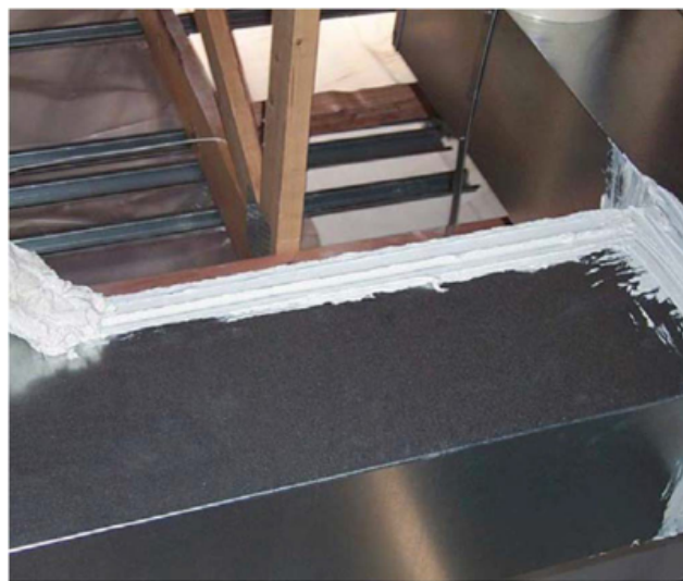
Metal ductwork sealed with mastic
