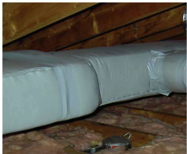
Sealed vapor retarder on attic ductwork
