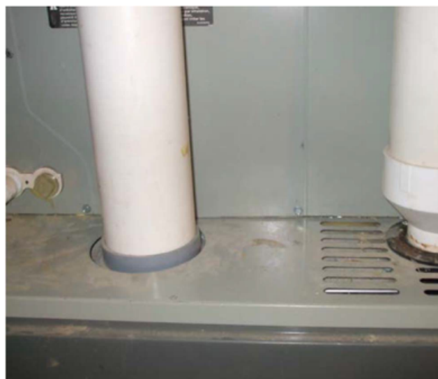
Air handler sealed with silicone caulk
