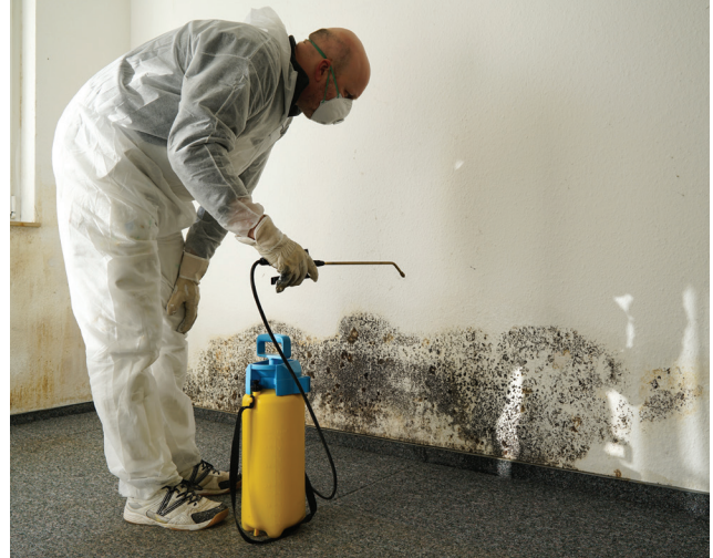
Mold on walls
